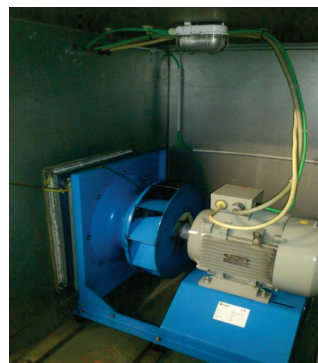
Before (Induction motor)
