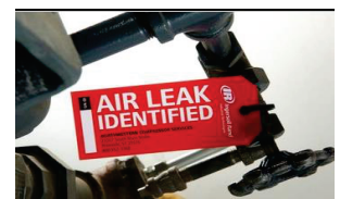
Figure 16 Red tag to air leakage point
