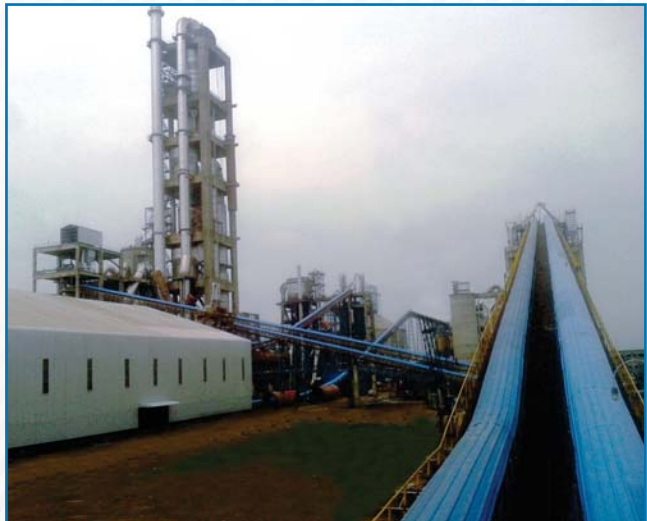
Limestone, Clinker Clay, Dolomite, Bauxite & Laterite Handling System at JK Cement
